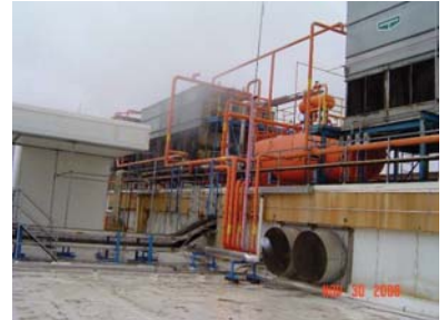
Evaporative Condensers & Receiver
