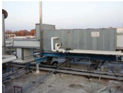
Freezer DX Coils & Air Handler
