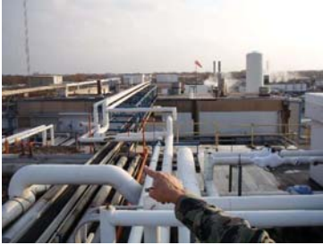
Refrigerant Piping & Pipe Rack
