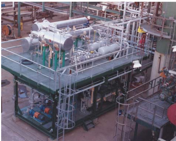
Evaporators, Absorbers & Pumps on Skid
