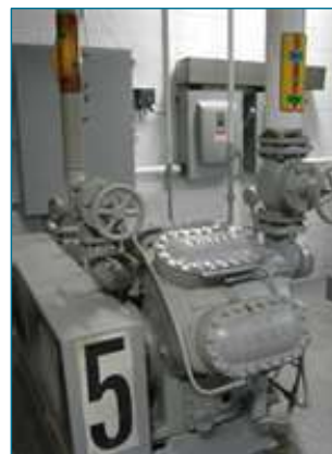
Vilter Ammonia Compressor
