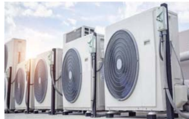
Decentralising plant resulting in part load inefficiencies.
