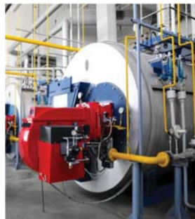
INDUSTRIAL TYPE GAS FIRED STEAM BOILER
