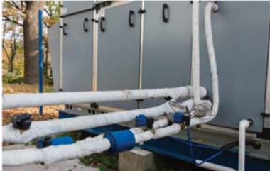
Poor insulation on heating and cooling pipework and AHU ducts.
